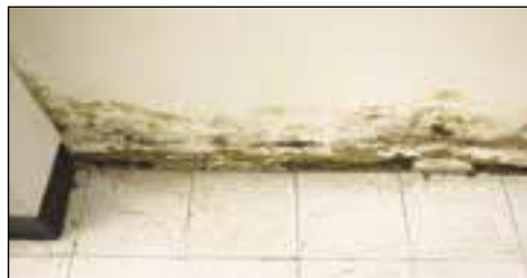
This is an example of damage and mold in the lower level of Austin's Law Enforcement Center. Mold has been sprayed to limit exposure, but it is still there.
